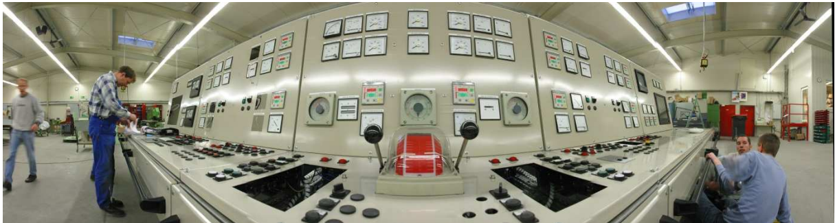
Control panel for the shipbuilding industry
